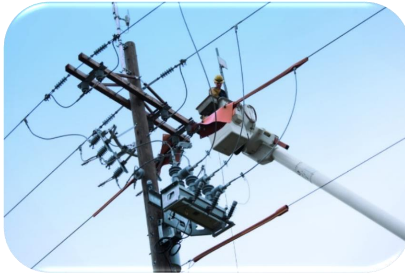
Distribution Recloser based PMU via protective relay
