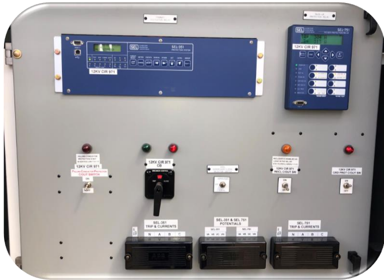
Substation Breaker based PMU via protective relay
