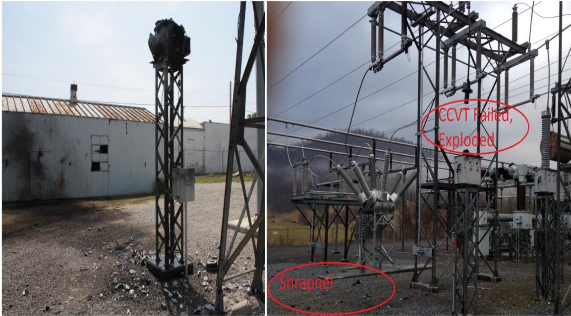
Example from AEP of failing CCVT in a substation
